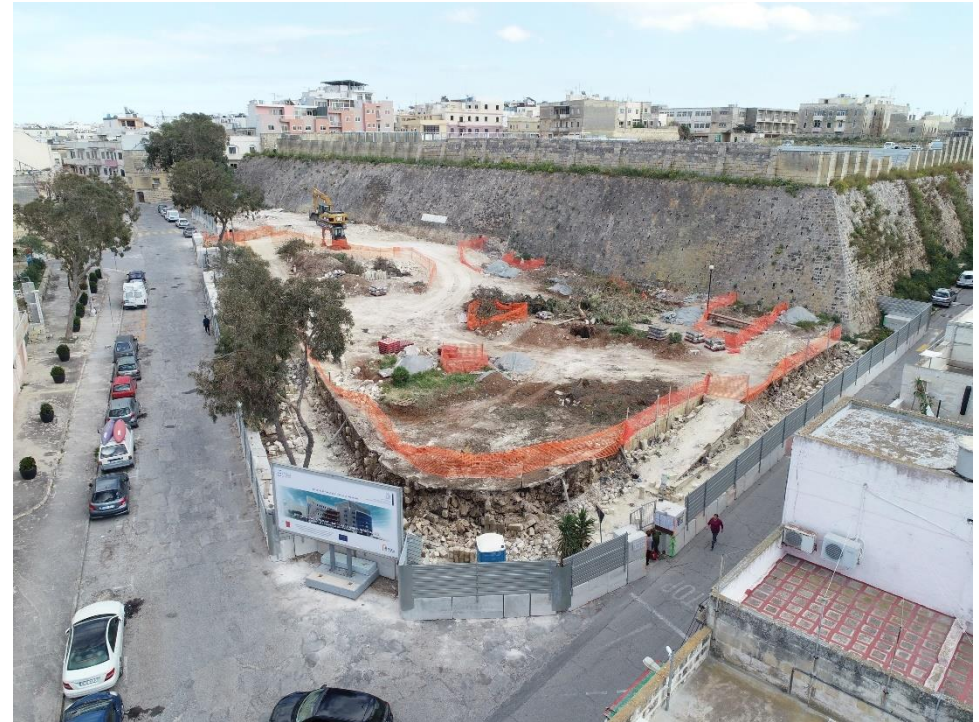
Demolition work, site clearance, preliminary access and hoarding at the Paola Regional Health Hub.
