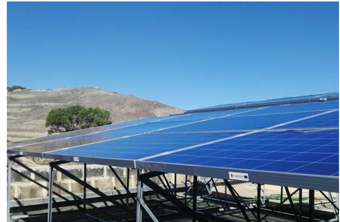
PVs installed at the OASI Foundation, generating 29.68KWp of renewable energy
