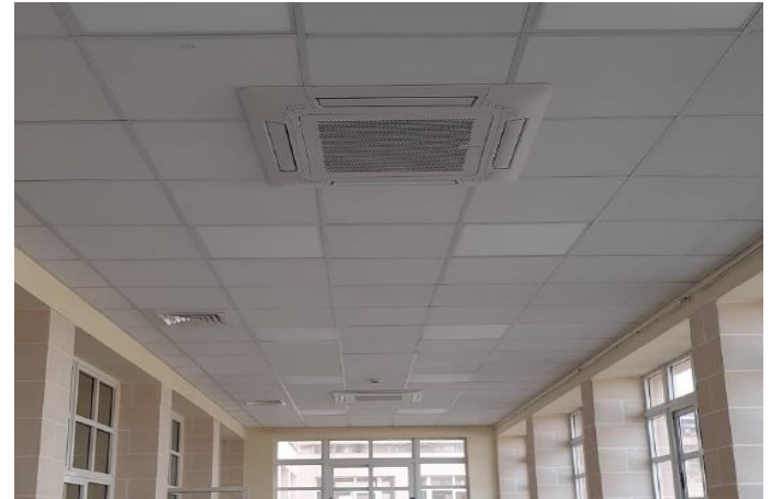
Energy Efficiency measures installed at Lourdes Ward, St Vincent de Paul Residence
