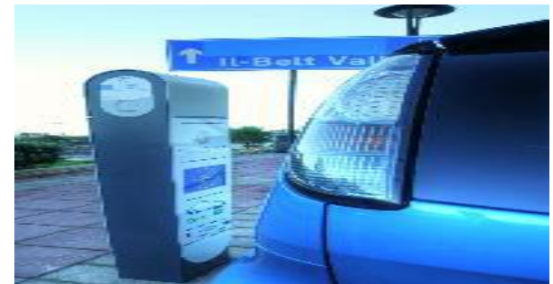
Installation of charging Pillars for electric vehicles
