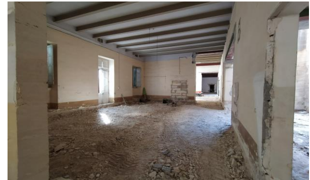
Hospice Malta Complex which will offer palliative care including facilities such as physiotherapy and occupational therapy rooms
