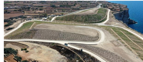
Aerial view of the Rehabilitated public area on former Wied Fulija landfill site
