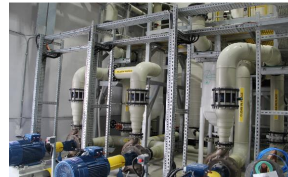
Part of the equipment installed at Gozo RO
