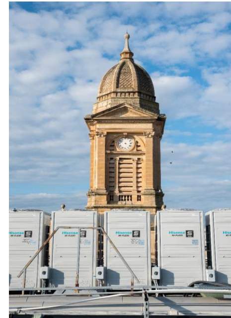
Energy efficient measures at St. Vincent's De Paul Residence (Elderly Home)
