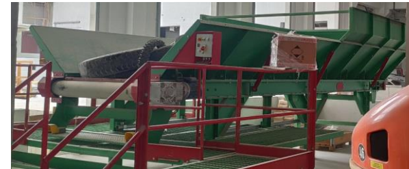
Tyre processing equipment installed at the MMRF site
