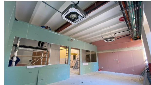
M&E works at the Hospice Malta Complex which will offer palliative care
