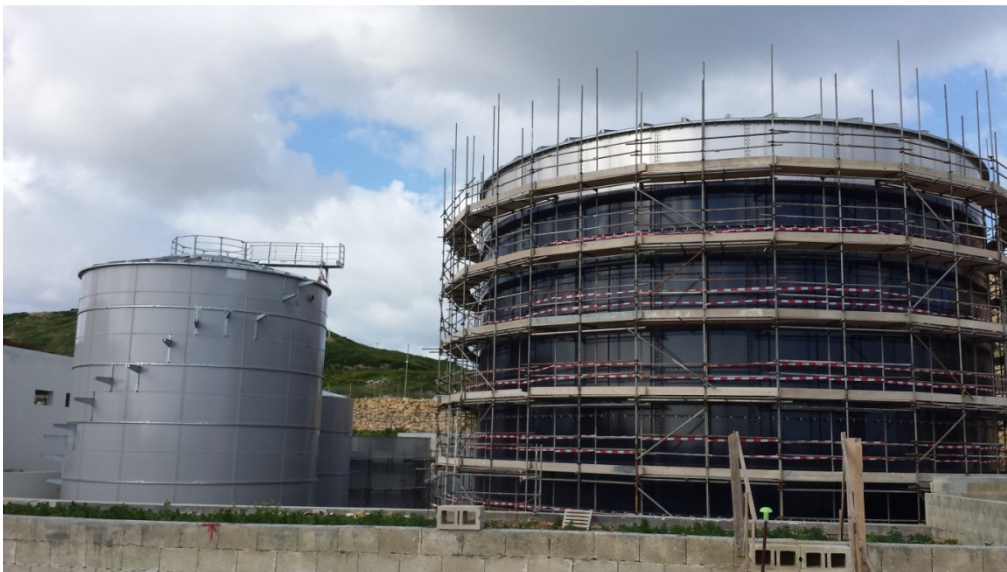
Figure 98 - Anaerobic Digestion Tanks
