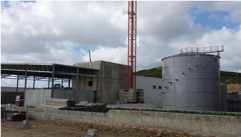
Figure 99 - Compost Shed and Dewatering
