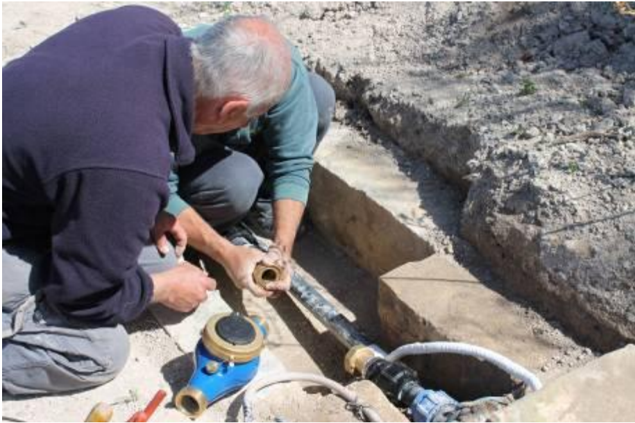
Figure 21 – Installation of smart water meters in the Chadwick Lakes area, limits of Rabat
