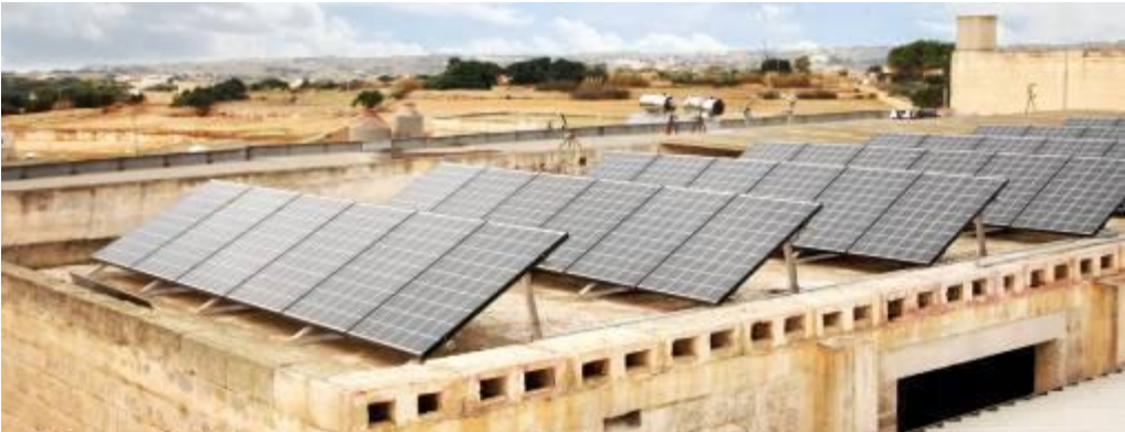
Figure 8 – Photovoltaic panels, financed through Measure 121
