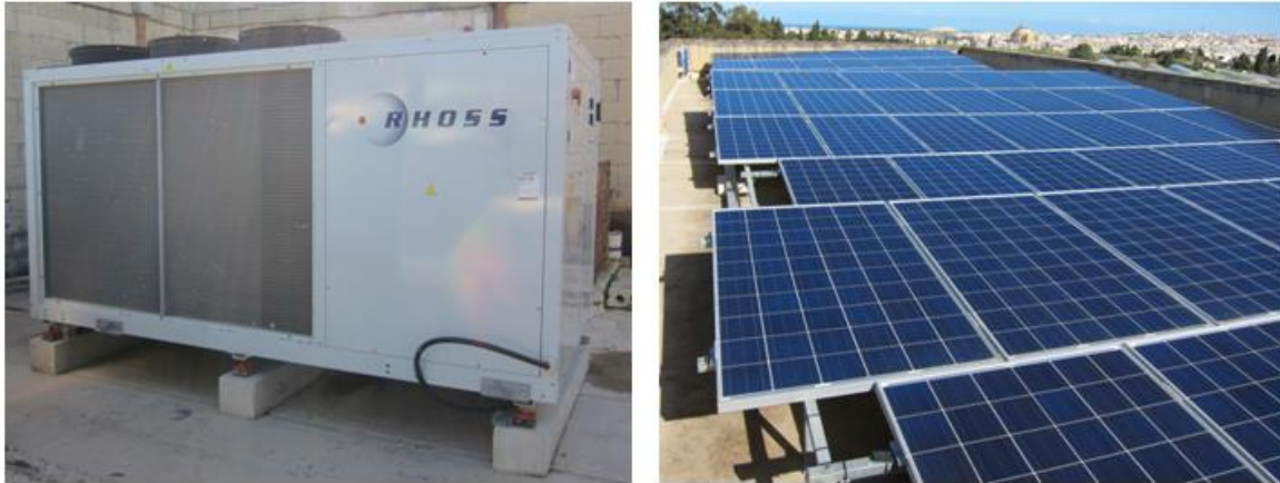
Figure 8 – Ciller and photovoltaic system installed by a local wine producer
