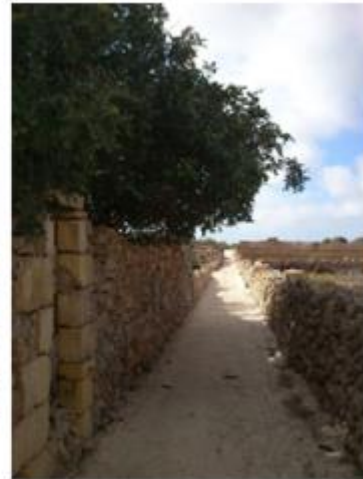
Figure 15 – Ministry for Gozo, part of M313 project: access to Santa Verna remains, before and after works
