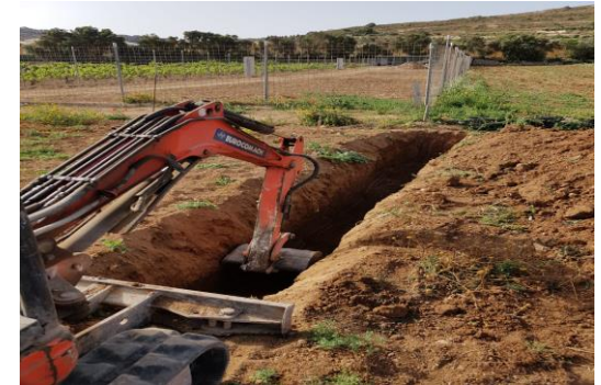
Ongoing works for the installation of a real time monitoring water network.
