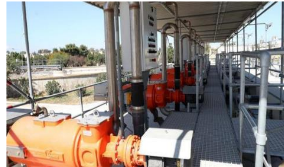
New water infrastructure at Sant'Antnin Wastewater Plant
