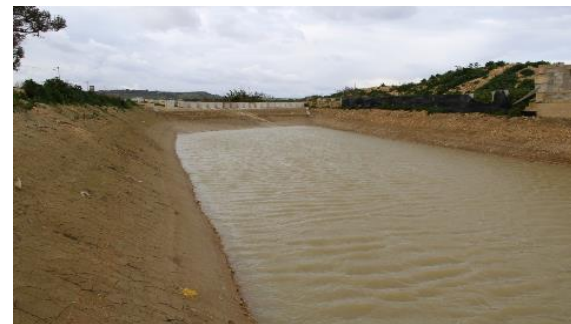
Ongoing works at the water basin 7 at Wied il-Ghasel under the Rainwiin Project
