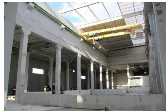
Loading bays with runner beams & part of canopy structure at the MMRF
