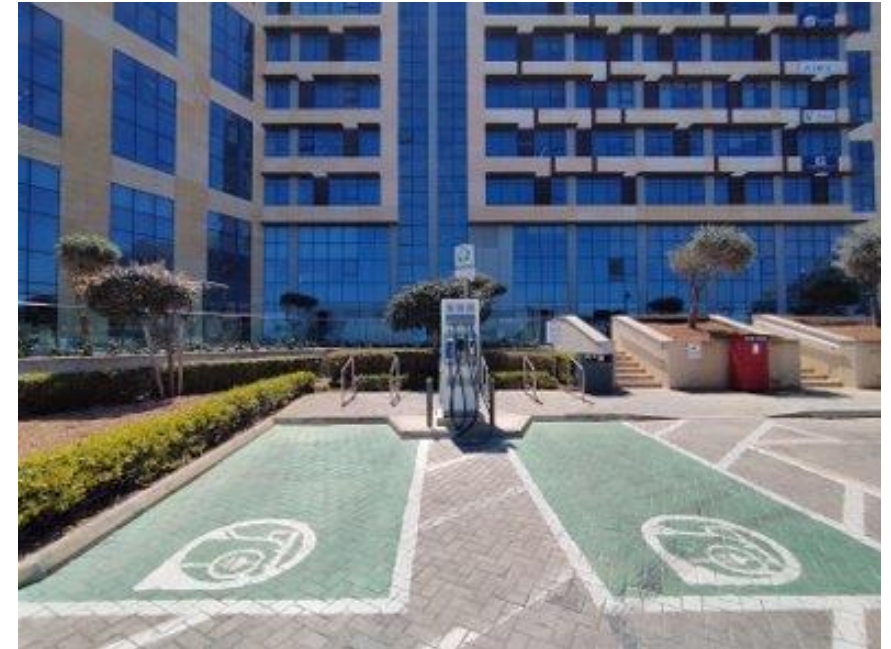
130 Charging Pillars installed.
