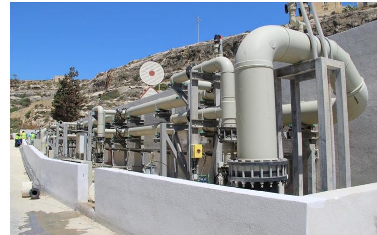
Wellfield piping at the Ffondoq RO Plant
