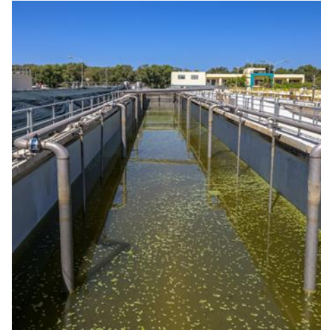
Sant' Antnin Wastewater Treatment Plant – Aeration lane retrofit with filter media
