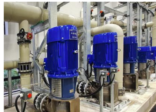
Hondoq RO – Seawater Feed Pumps
