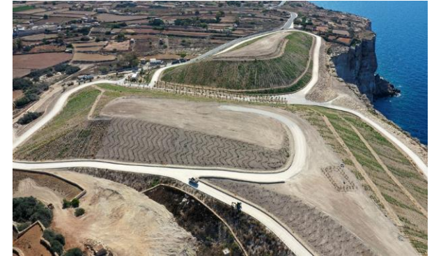
Aerial view of the rehabilitated area on the former Wied Fulija landfill site
