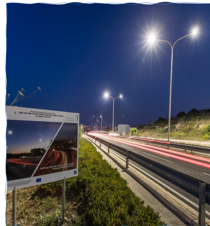
Upgrading of streetlighting with energy efficient LED lanterns together with the installation of a light management system
