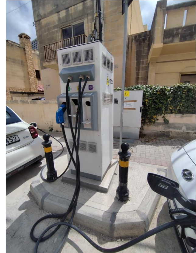
Current Charging Pillar Infrastructure
